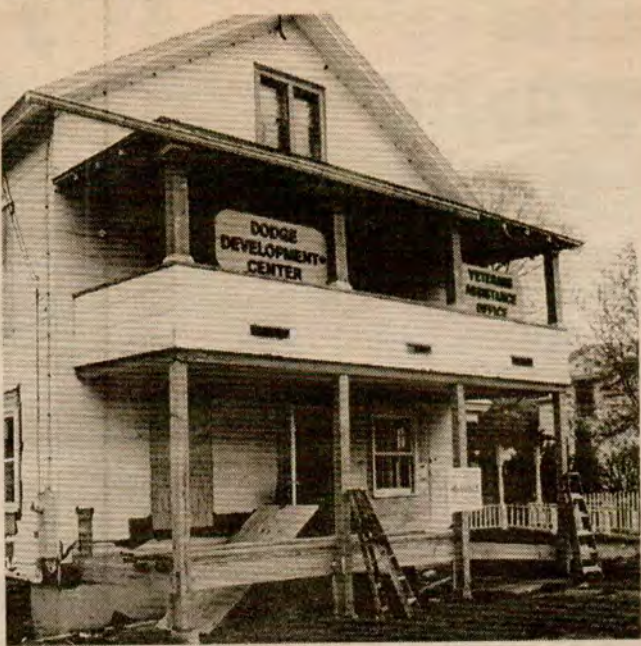
Renovations continue at the VVA's Dodge Development Center in Rutland Bob Perry photo
